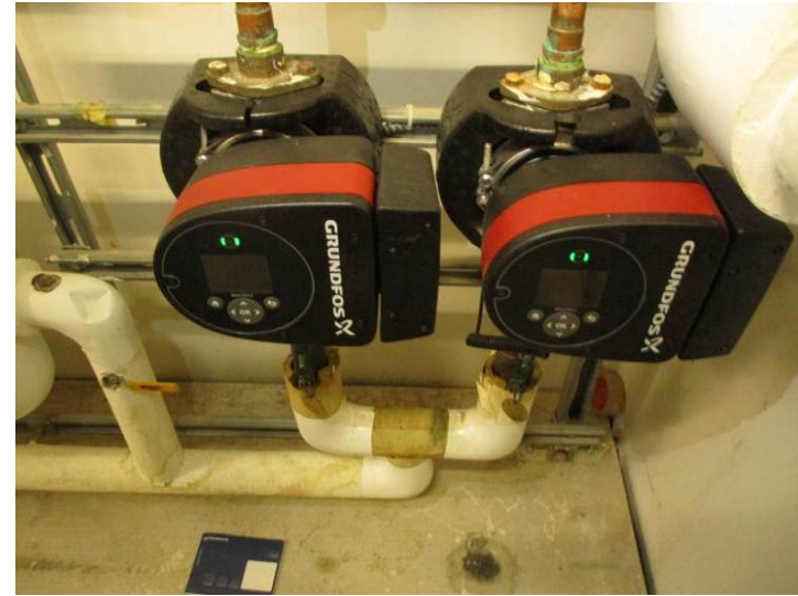
This DHW system features two in-line, Grundfos MAGNA3, high-efficiency, 1/8-hp, stainless-steel, delivery and return pumps and a single Leonard thermostatic mixing valve.
