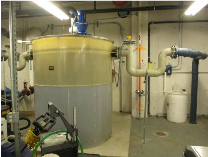
An acid neutralizing system serving the science labs is also located inside the large ground-floor boiler room.
