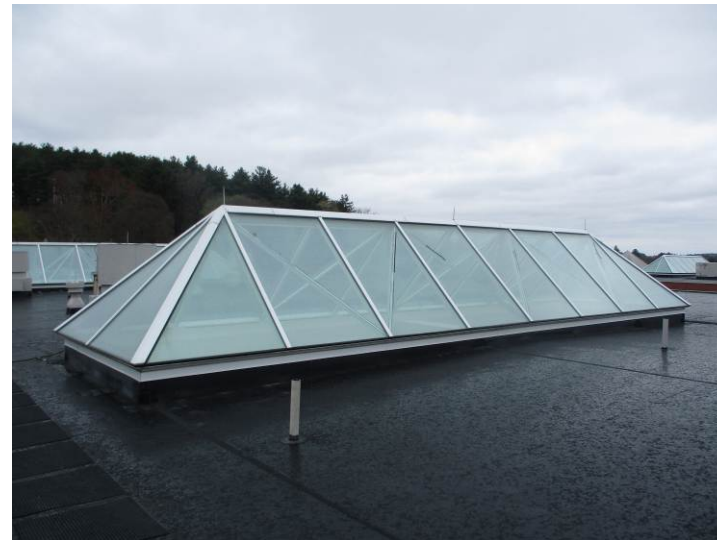
The large aluminum-framed skylight assemblies illuminating the corridors and various rooms at all three sections are reportedly in need of near-term sealing/maintenance/refurbishment.
