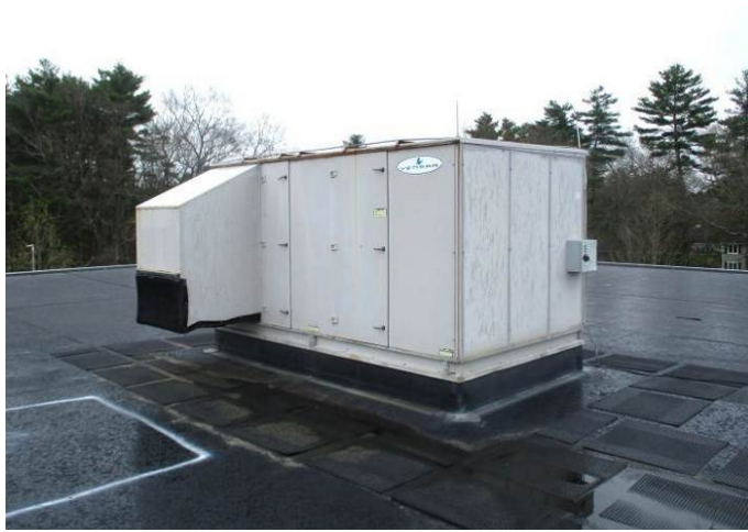
Thirteen rooftop-mounted Venmar ERV's provide fresh and conditioned air to various other sections of the building.
