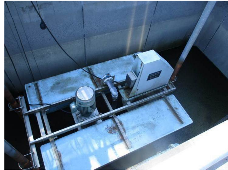
The tanks feature a mix of exposed and submerged pumping systems.
