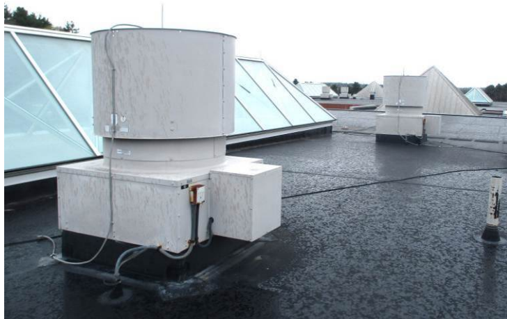
Each building section (A, B, and C) also features four large Greenheck, 20,000-cfm, up-blast smoke control fans that are controlled by the central fire alarm system.
