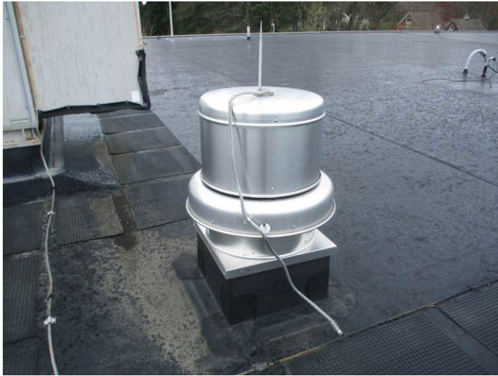
Additional localized building ventilation is produced by a series of smaller rooftop-mounted (all replaced in 2023) and interior-mounted in-line centrifugal exhaust fans.
