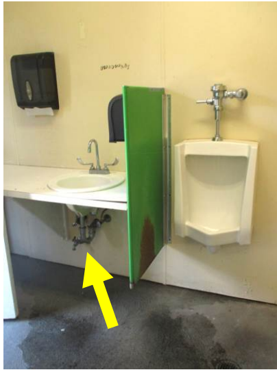
The men's and women's fieldhouse restroom sinks lack compliant piping insulation; and the men's room urinal needs to be lowered to compliant height. The rim should be positioned no higher than 17-inches above the floor.
