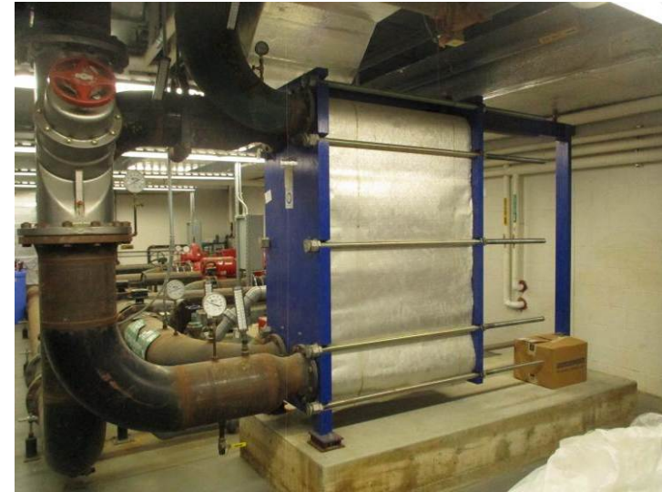
A large (319 plate) Mueller plate and frame heat exchanger transfers the collected heat within the service-water “closed” loop to the condenser-water “open” loop which is then delivered to the cooling tower for release. This separation protects the water-source heat-pumps from potential contamination.
