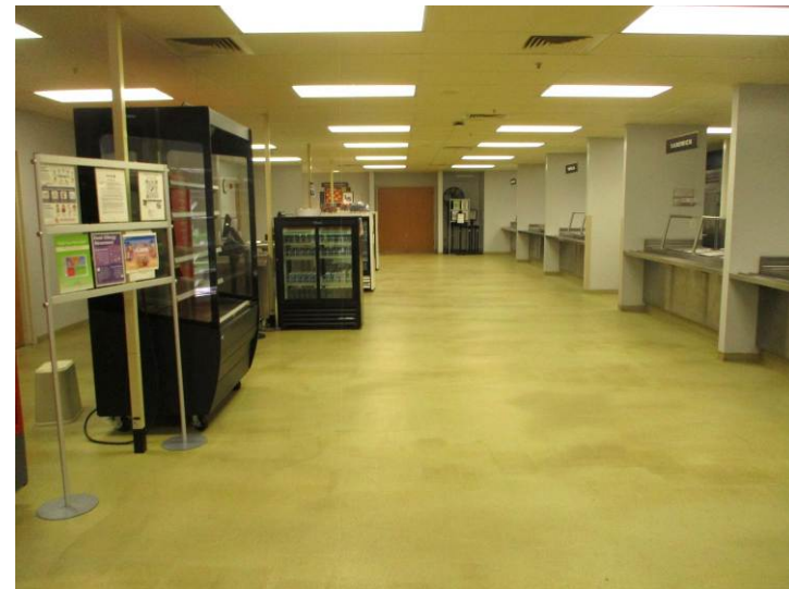
The cafeteria service area features a roller-applied epoxy-coat flooring that will be stripped down to the original concrete in the near term. The epoxy traps dirt and is difficult to keep clean.
