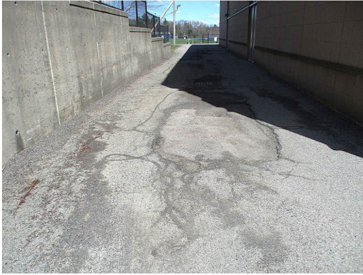
Significant asphalt deterioration observed at the east side of the C block will be addressed in the near term (per management)
