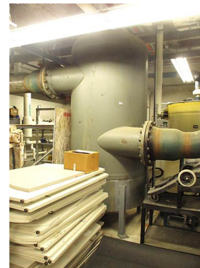
A large Bell & Gossett, 700-gallon air separator removes both air and dirt from the HVAC system to ensure optimal heat transfer, corrosion prevention, and noise reduction.
