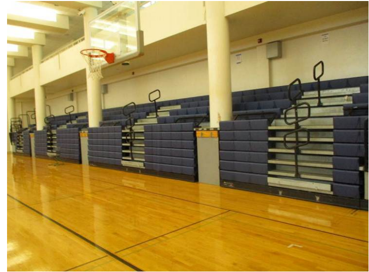
The electric (motorized/telescopic) bleachers reportedly date to the original 2004 construction but remain in generally good current condition.
