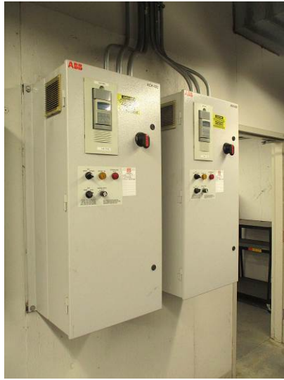
The cooling tower fan motors are controlled by individual wall-mounted, ABB ACH400, 20-hp, variable frequency drives that are located inside the adjacent boiler room.
