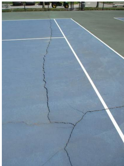
The cracking is extensive and non-repairable. A near-term full replacement of the base-course and surface is needed.
