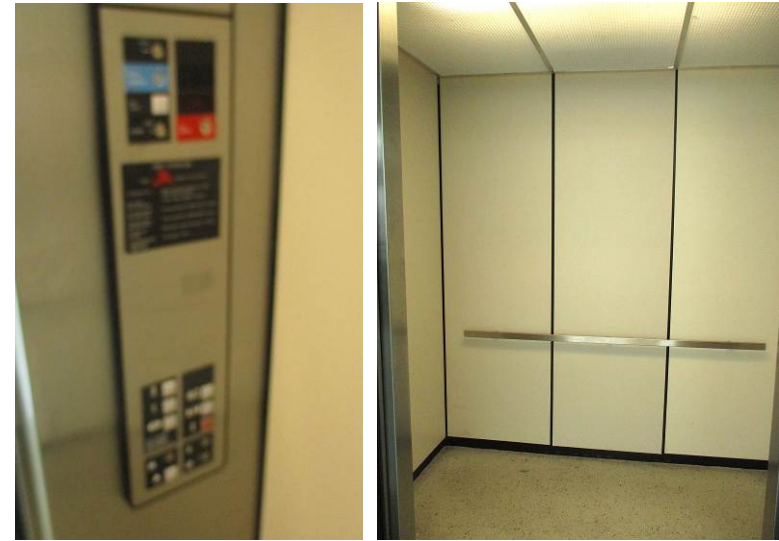
The A-section elevator cab finishes, door/floor buttons, and single access door.
