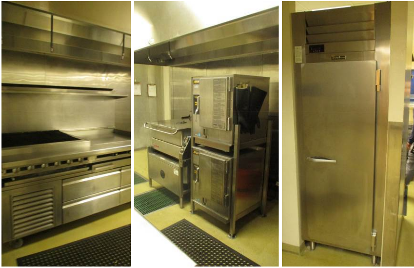
The cafeteria kitchen features a large collection of commercial food preparation, cooking, heating/warming, refrigeration, and dishwashing/sterilization equipment that all varies in age.
