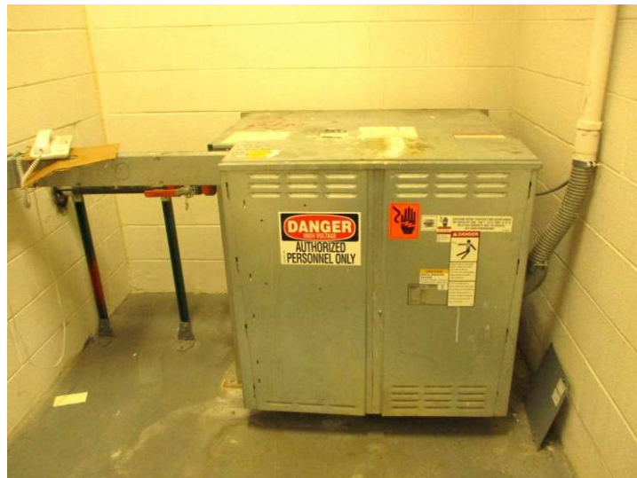
The B-section features an Otis four-stop hydraulic elevator system with 40-hp submerged-pump hydraulic power unit and machine-mounted solid-state controller.
