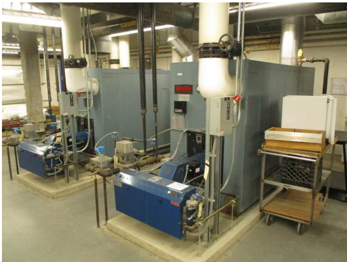
The majority of the interior spaces are heated and cooled by a four-pipe water-source heat-pump HVAC system. The service optimal water temperature range (70°- 90°) is maintained by a pair of Smith Series 28A, 13-section, 2,867-mbh, natural gas-fired, commercial, cast-iron, hot-water boilers.
