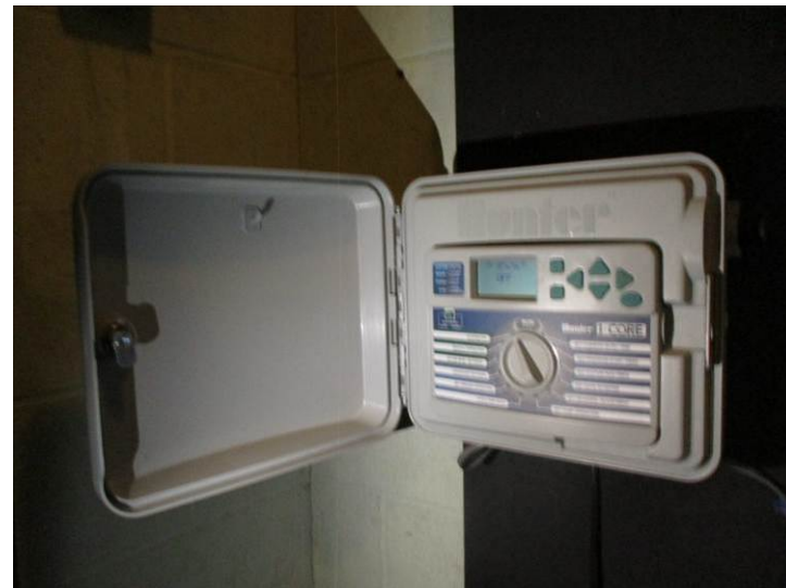
A large Hunter control panel (located inside the former boiler plant building) controls the irrigation system extension that serves the softball field located at east end of the property.
