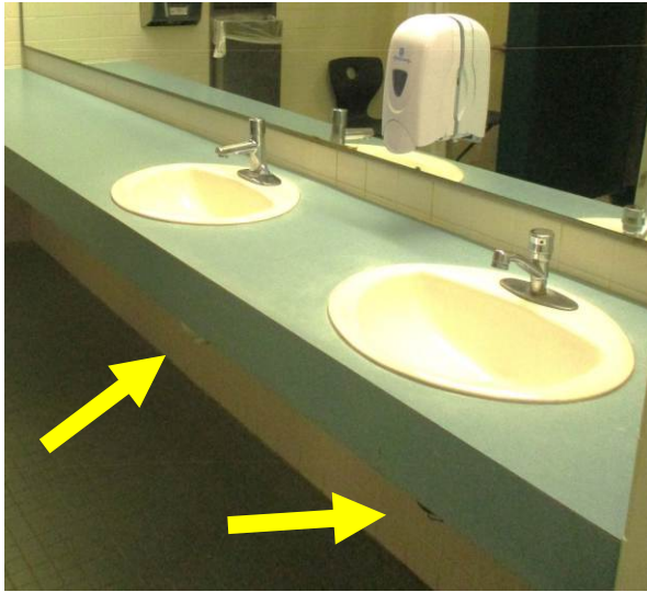
One sink at the shower-area sink-counters has covered piping, the other does not.
