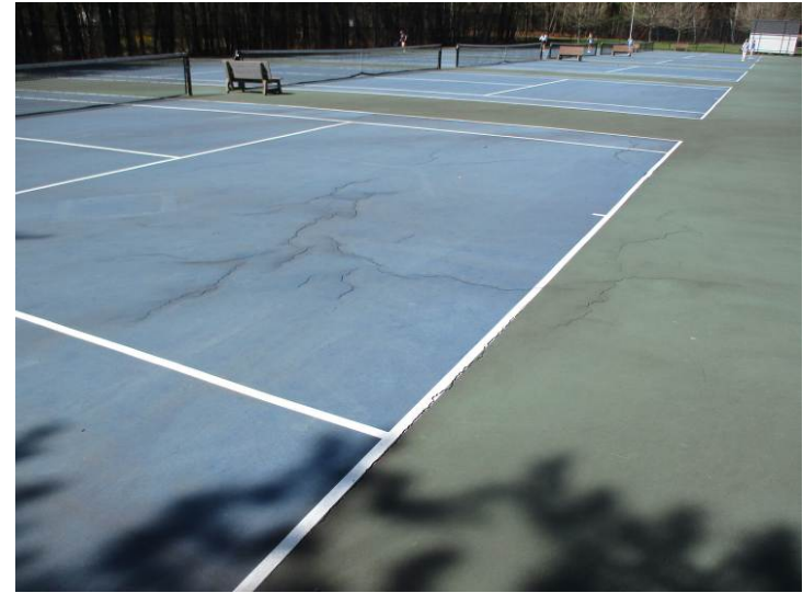
The asphalt/acrylic-surface tennis courts were repainted in 2021 but exhibit widespread age-related cracking.
