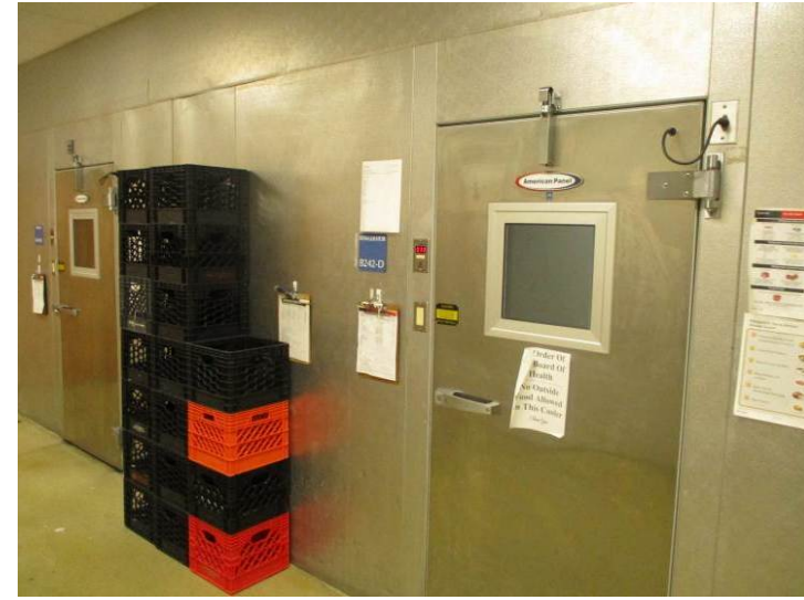
The kitchen also features four commercial walk-in coolers (two refrigeration, two freezer) with rooftop-mounted condensers.
