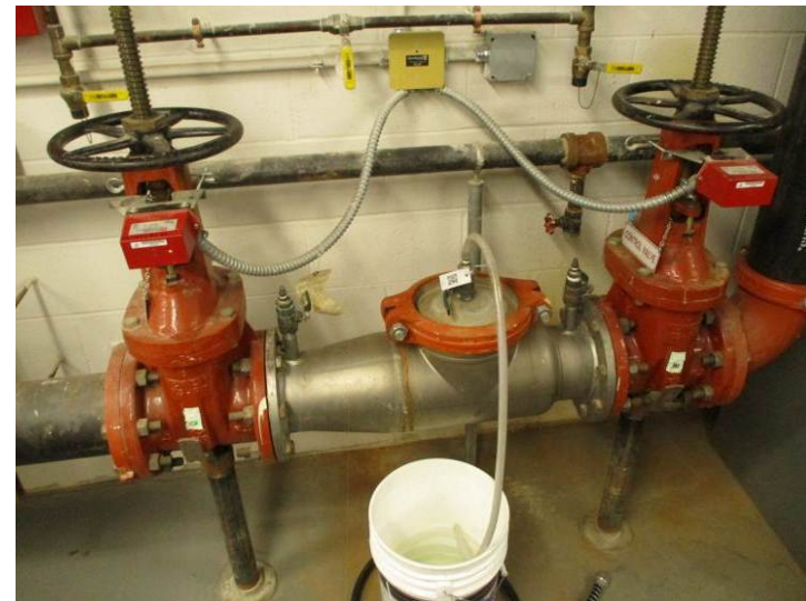
The building is protected by a full-coverage, street-pressure driven (no fire pump) fire-suppression sprinkler system with backflow preventer in place (located inside the boiler room).
