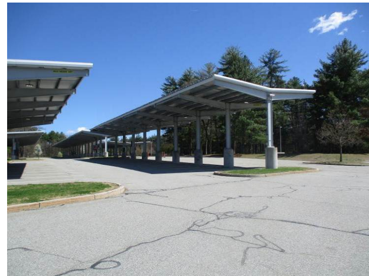
The upper parking lot features a series of steel-framed carport structures supporting a large photovoltaic system that is owned and maintained by the installation contractor. In exchange for the power generated, the school receives a beneficial fixed 11-cent per kWh usage rate for twenty years (2015-2035).
