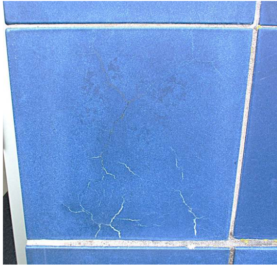
The simulated blue tile is actually a glazed masonry veneer that is developing visible age-related cracking.
