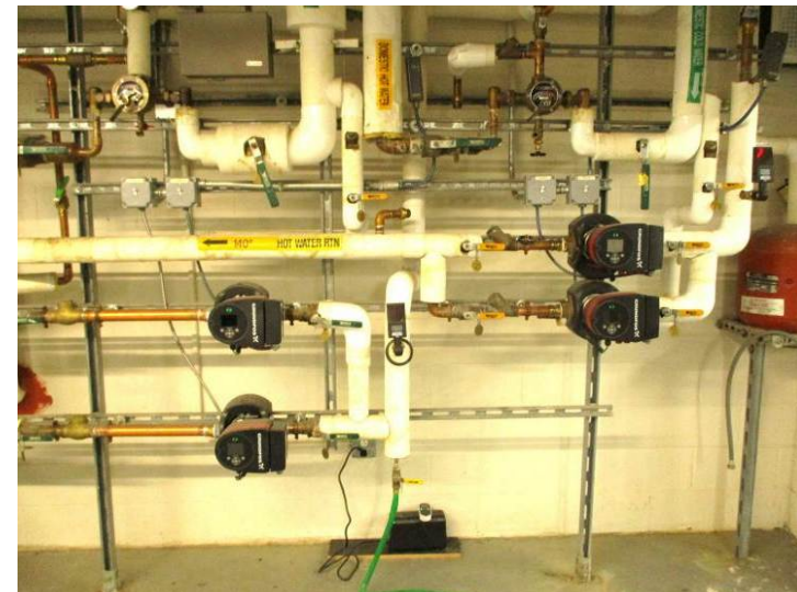
The DHW system also features four in-line Grundfos MAGNA3, high-efficiency, 1/8-hp, stainless-steel, delivery and return pumps, and two Leonard thermostatic mixing valves.
