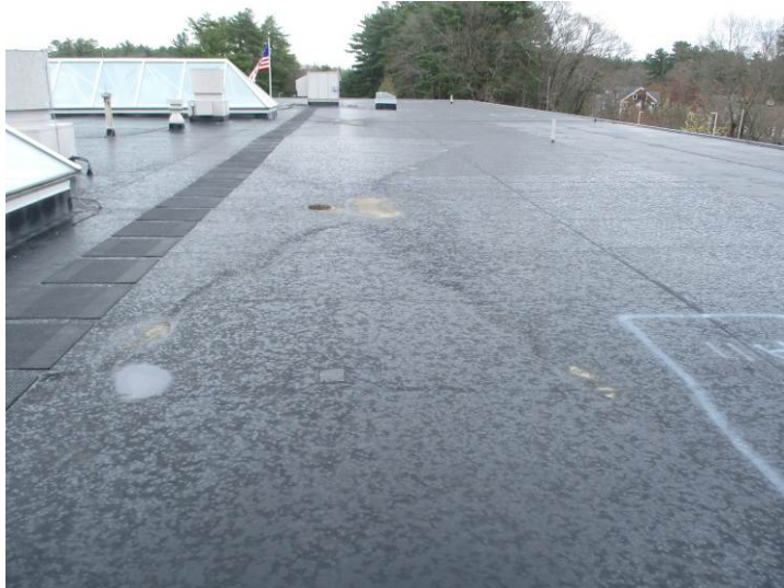
Typical single-ply EPDM membrane roof covering at all three sections. All three coverings date to the original 2004 construction and are in need of near-term replacement.
