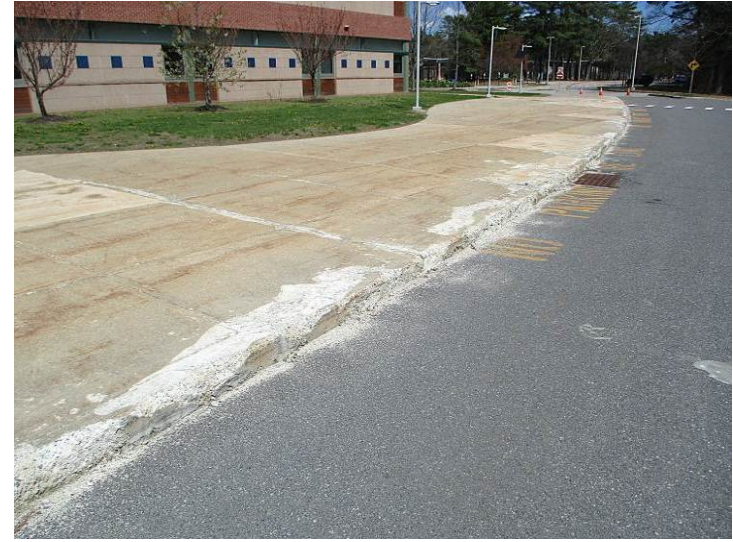
The significant salt/snow-melt related concrete flatwork deterioration at the front/main and auditorium entrance plaza will also be addressed in the near term.
