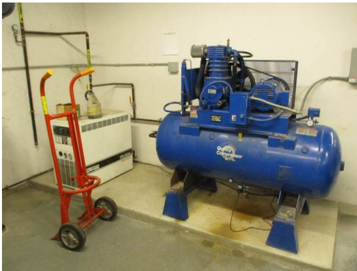
The pneumatic shop tools are powered by a Quincy 10-hp, 30-40-cfm, 120-gallon, two-stage, heavy-duty, reciprocating air compressor with adjacent Airtek refrigerated air dryer.
