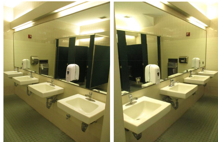
The toilet-area sinks at the boy's locker-room (left) and girl's locker room (right) all have exposed/uncovered piping.
