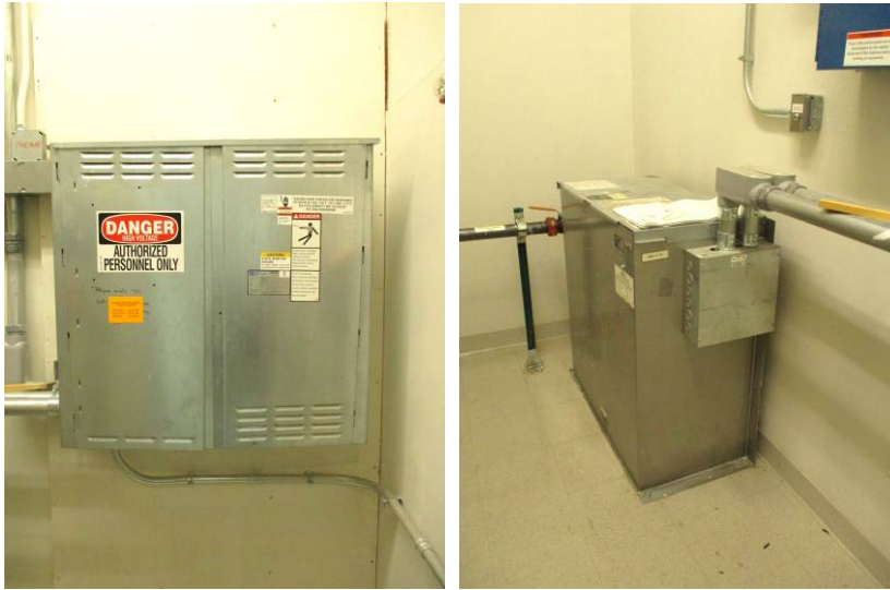
The A-section features an Otis three-stop hydraulic elevator system with 25-hp submerged-pump hydraulic power unit and wall-mounted solid-state controller
