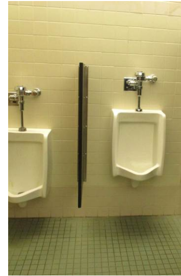
The multi-stall restrooms feature one standard-height urinal and one accessible-height urinal (which is ADA acceptable).
