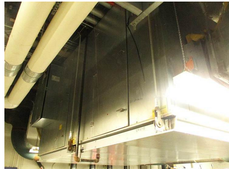
Three interior, ceiling-mounted, Venmar energy-recovery ventilators (ERV-1, ERV-2, and ERV-8) utilize the energy in the stale building exhaust air to precondition (humidify or dehumidify depending on season) the incoming fresh air.
