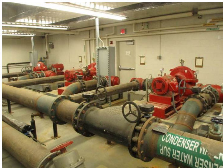
The condenser water (cooling tower) loop is circulated by three base-mounted horizontal split-case pumps with 30-hp motors.
