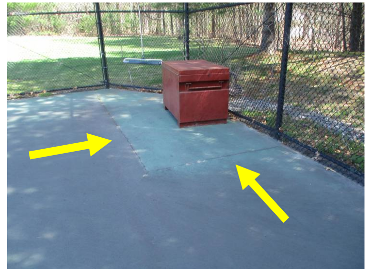
The collapsed northeast-corner was repaired, but is cracking and settling again. These issues are most likely related to the location of the courts which appears to be at a low-point of the property where drainage water migrates and settles.
