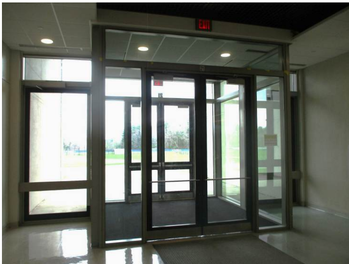
The lower (ground-floor) level of the Section C features several large, oversized, aluminum and glass doors that exhibit visible weight-related alignment issues requiring ongoing maintenance and repairs (per management).
