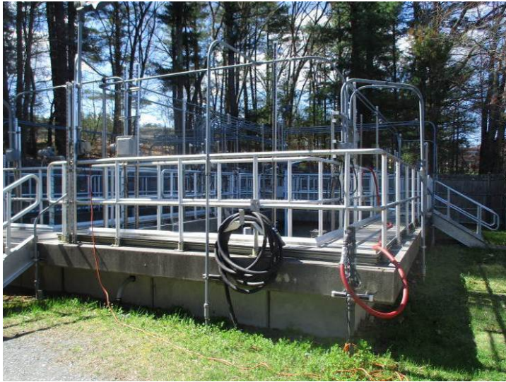
The property also features a sequencing batch reactor (SBR) style wastewater treatment facility (featuring various open/exposed and below-ground influent, reactor, mixing, aerating, and settling tanks) that was newly constructed in 2004.
