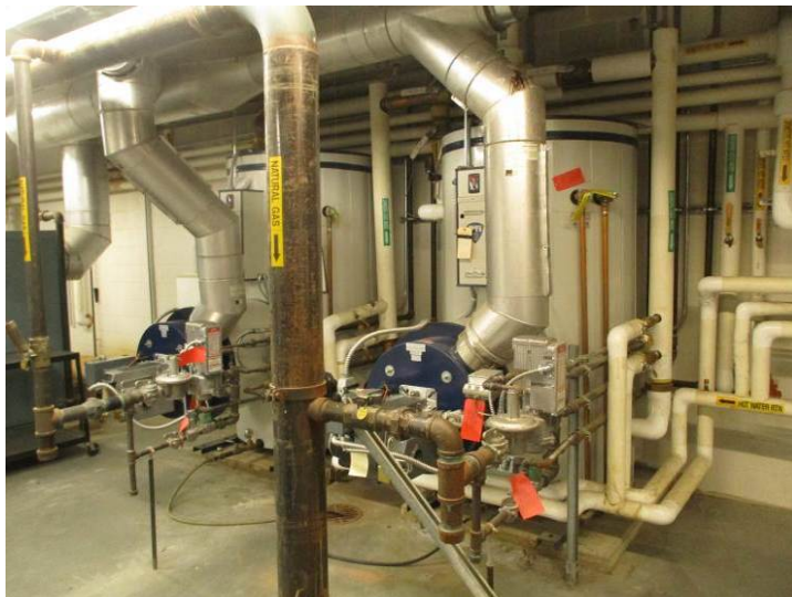
Domestic hot water for the majority of the building is produced by a pair of PVI AquaPLEX Turbopower, 400-gallon, 1,200-MBH, 1,200 gph, natural gas-fired, stainless-steel, commercial storage water heaters that vary in age (installed in 2016 and 2019).
