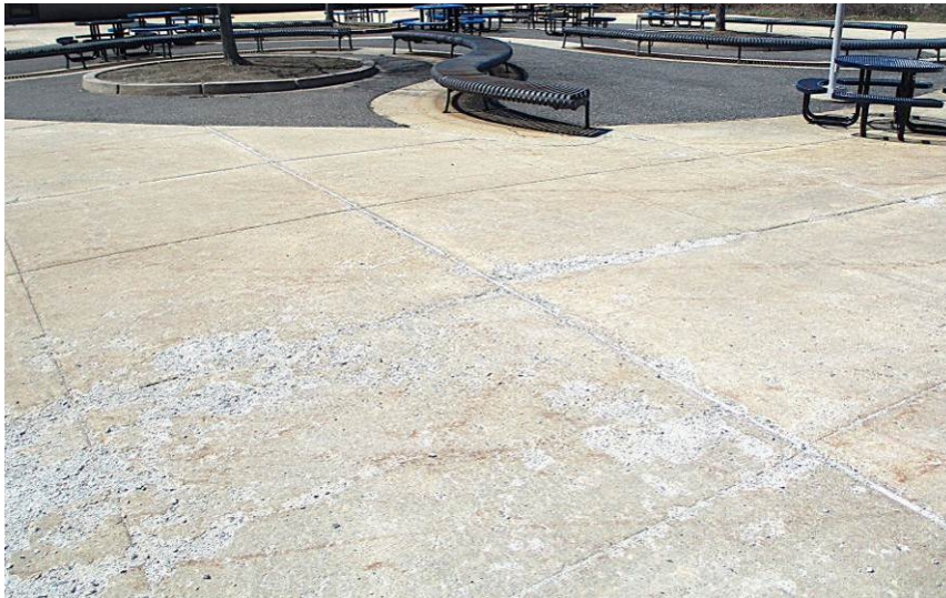
Similar concrete surface deterioration is developing at the cafeteria plaza.
