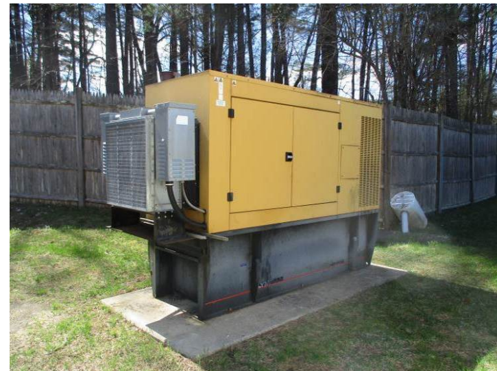
The facility also features a dedicated Olympian 150-kW diesel-powered standby emergency generator with sub-base fuel oil storage tank that dates to the 2004 system installation.
