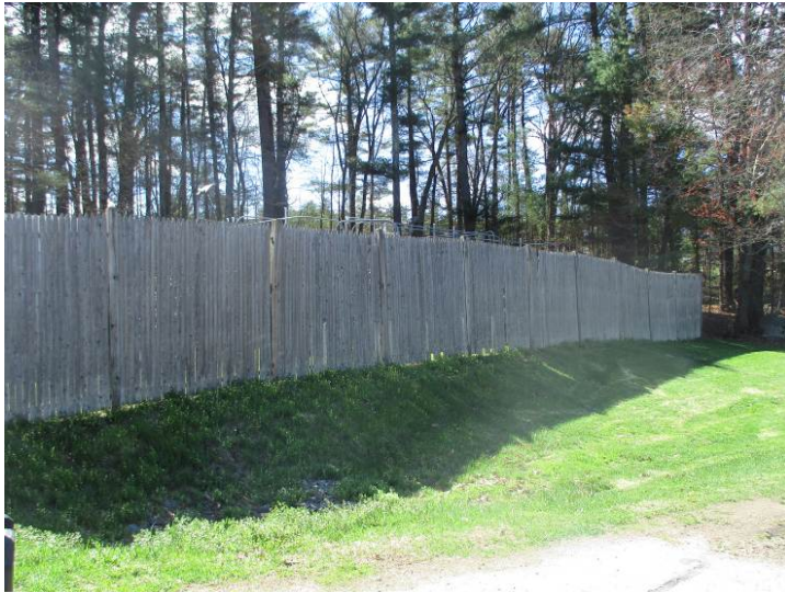
The visibly older, ageing, wood-stockade perimeter fencing at the wastewater treatment facility is in need of near-term replacement.
