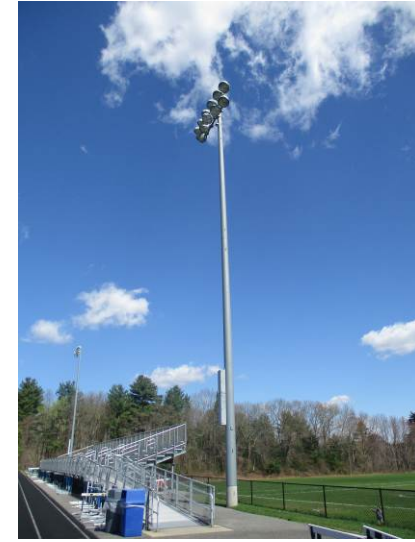
The four large sectional galvanized-steel poles (two on each side of the field) and large sodium discharge field-lighting fixtures were all newly installed in 2012.
