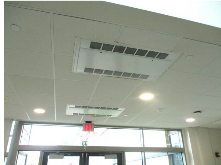
The wall-mounted and ceiling-mounted, recessed electric unit heaters that provide supplemental heat at the various upper and lower-level entrances and stairwells are all in need of near-term replacement (per management).
