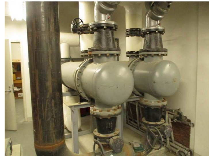
The boiler-water heat is transferred to the service water loop via two adjacent Bell & Gossett, 2,700-mbh, 300-gpm, shell-and-tube-style heat exchangers.
