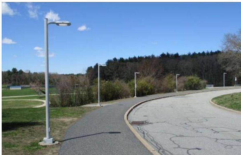
The parking lots, roadways, and adjacent walkways are illuminated by a series of pole-mounted energy-efficient LED surface lighting fixtures that were all newly installed in 2015.
