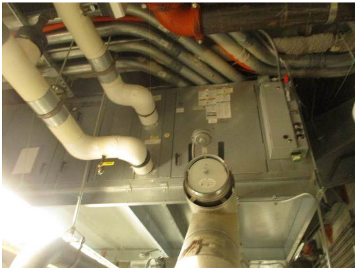
Fresh and tempered air makeup-air for the lower-level locker rooms is produced by a ceiling-mounted, McQuay, 7,200-CFM, 556-MBH, makeup air unit (located inside the boiler room).
