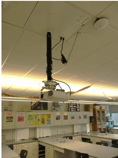
The ceiling-mounted digital classroom projectors reportedly vary in make, model, and age throughout the building.
