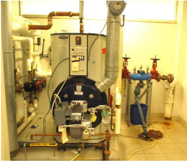
A smaller 150-gallon, 399-mbh, 400-gph, PVI water heater produces DHW for the various science classroom sinks (installed in 2018).
