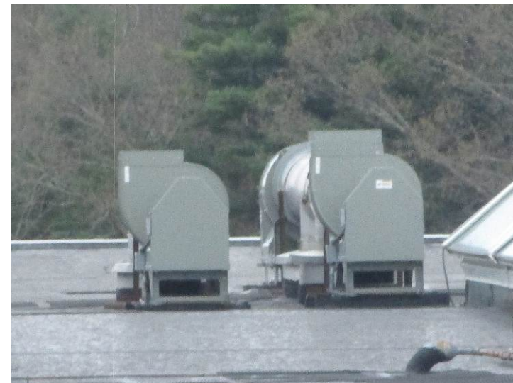
Three rooftop-mounted 2,750-cfm, 2,810-cfm, and 4,050-cfm belt-driven, upblast utility blowers produce the exhaust needs for the large commercial kitchen at the section B cafeteria.
