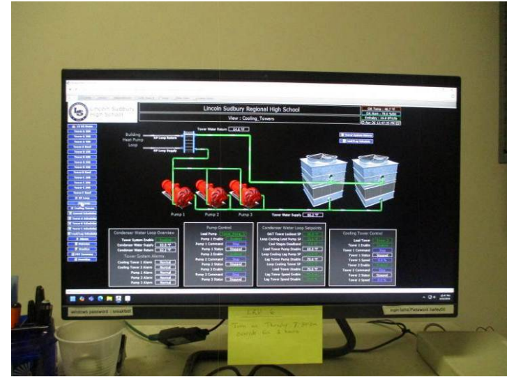
The entire HVAC system is monitored and controlled by an energy management system that utilizes a mix of hardware endpoints and software to monitor, analyze, and optimize equipment/system operation and energy consumption.
