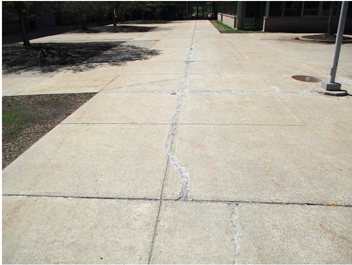
Similar concrete flatwork deterioration observed at the student entrance plaza (adjacent to the cafeteria plaza).
