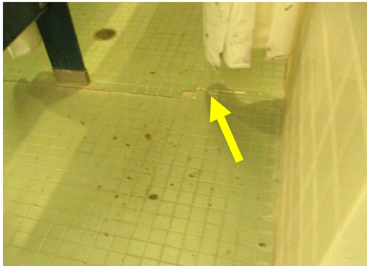
Ageing, cracked, damaged, tile flooring observed in the boys locker room shower area.
