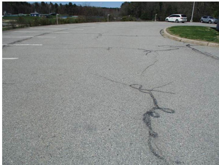
Typical drive-aisle and parking stall asphalt-surface conditions observed at the upper/main parking lot.
