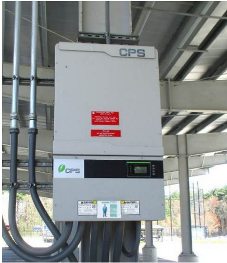
The photovoltaic system also features 35 post-mounted 28,000-watt grid-tie inverters that are also owned, maintained, and will be replaced when-needed by the installation contractor.
