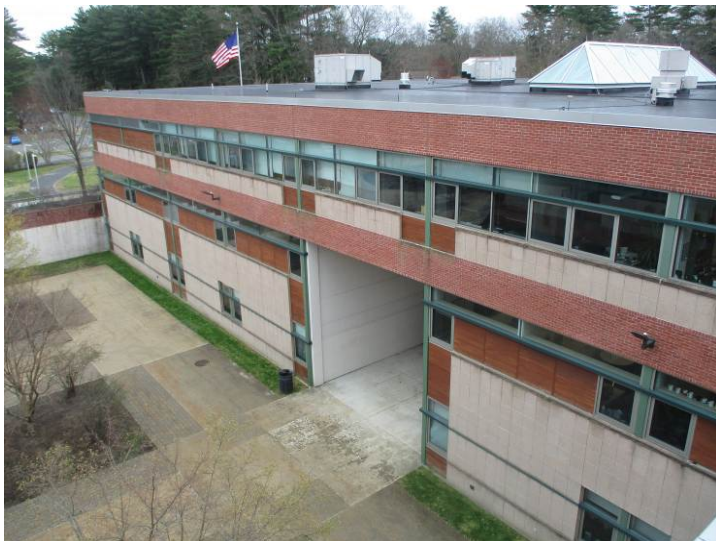
The north-facing elevation of Section A at the east-facing student entrance courtyard. The aging, deteriorating joint caulk (between dissimilar cladding materials) and the window perimeter caulk reportedly date to the original 2004 construction of the building and is in need of very near-term replacement.
